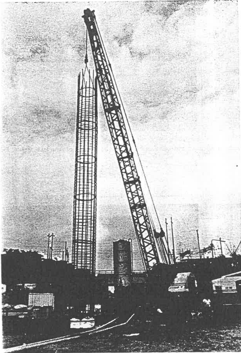
Fig. 5 - View of the setting in operation of a preload cell, which is jointed to the steel reinforcement.
